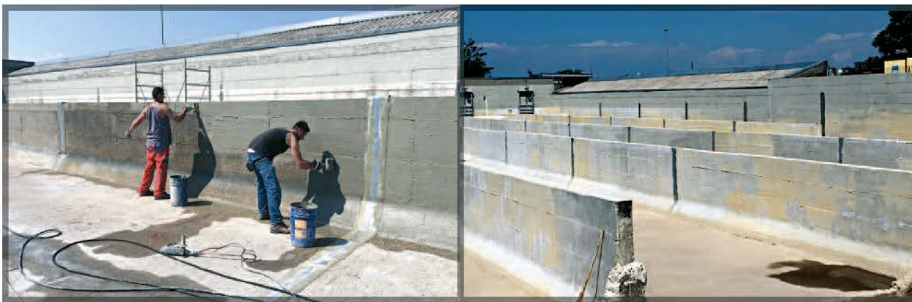
Vasca geotermia, ENEL GREEN POWER, Larderello (PI)
